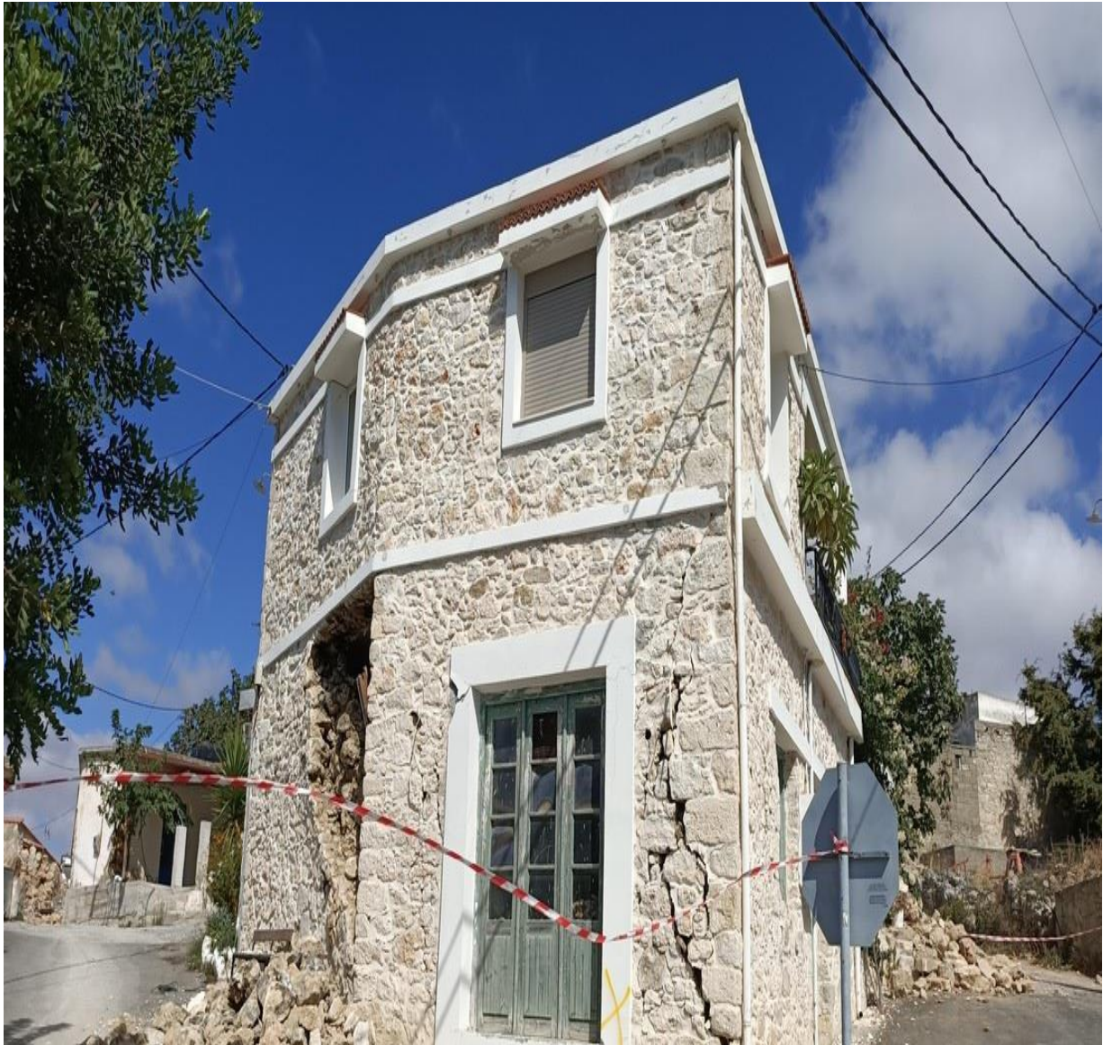
Figure 6 – Damaged house on the island of Crete in Greece as a result of the Arkalochori earthquake in 2021.
