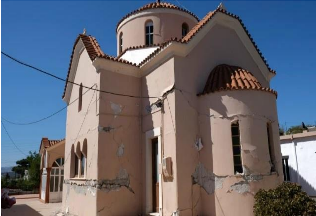
Figure 11 – Damaged Greek Orthodox church on the island of Crete in Greece as a result of the Arkalochori earthquake in 2021.
