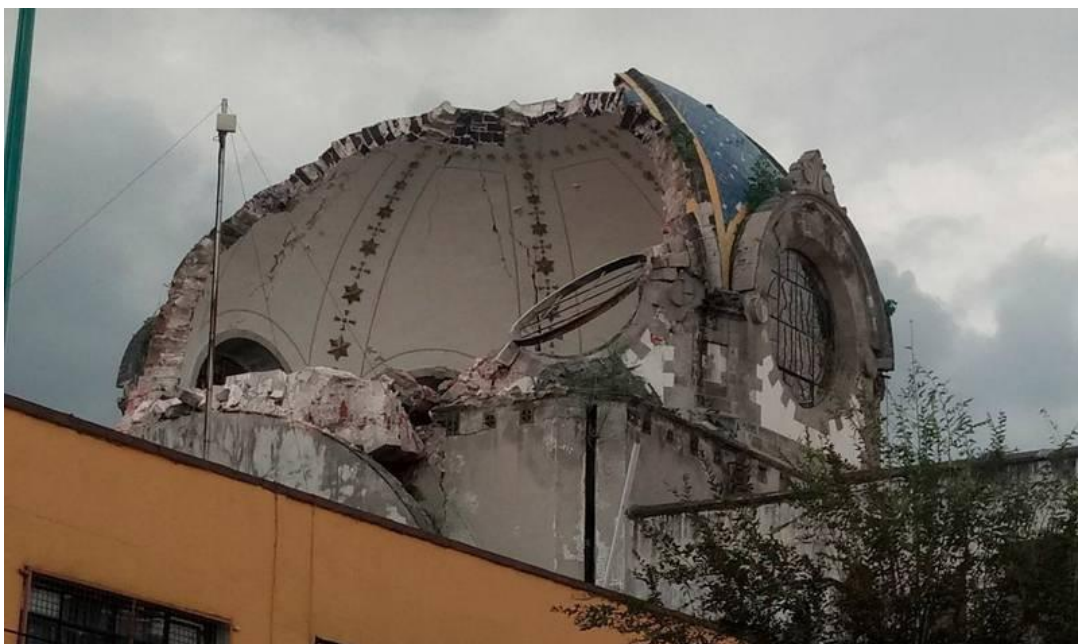
Figure 12 – Damaged dome of Catholic temple “Sanctuary of Our Lady of the Angels” as a result of the 2017 earthquake in Mexico City, Mexico.
