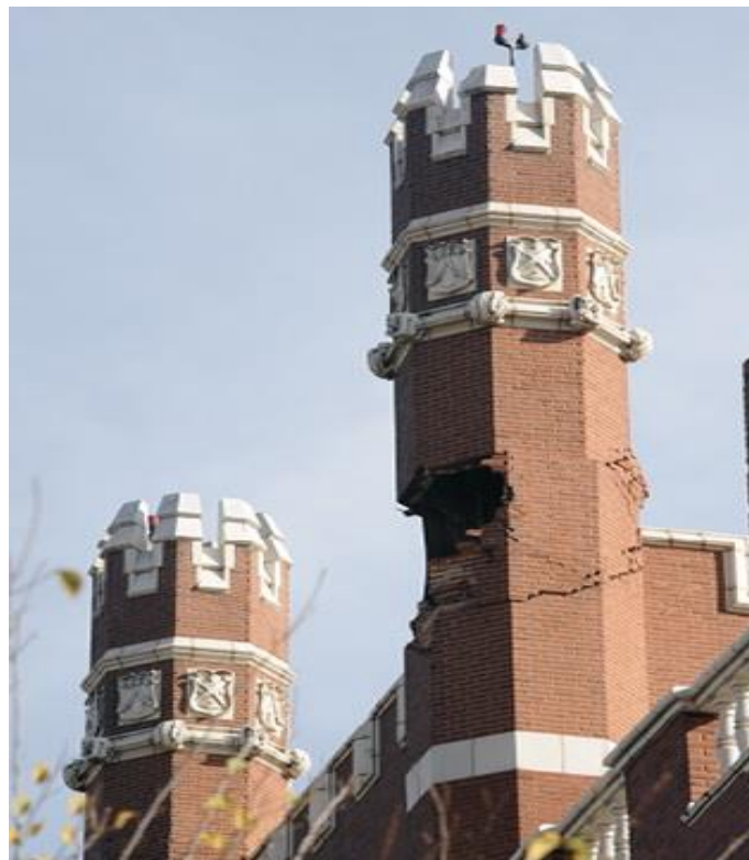
Figure 8 – Damaged Benedictine Hall turret at Saint Gregory University in Shawnee, Oklahoma USA, in the 2011 earthquake.
