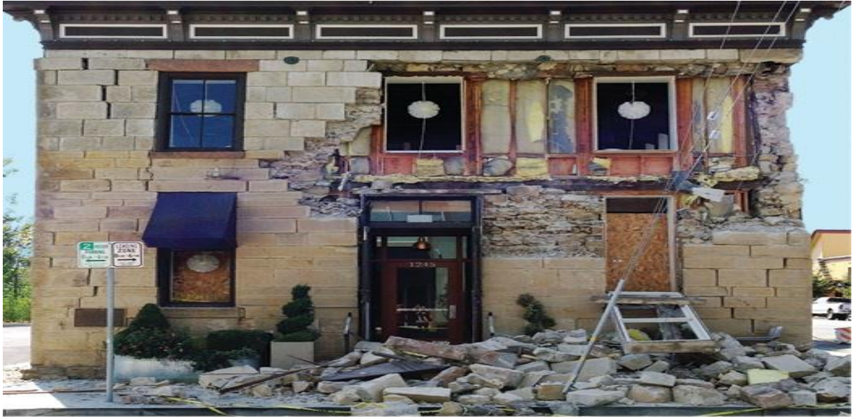
Figure 7 – Damaged old masonry building built in 1875, during the earthquake in South Napa, California, in 2014.
